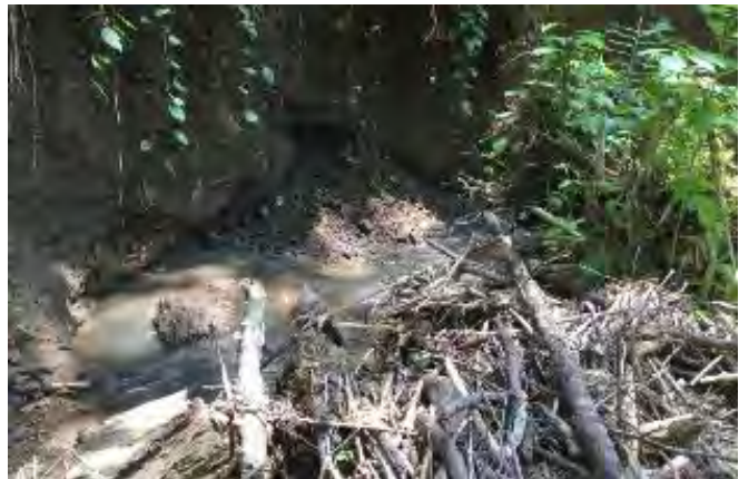
Plate 3.21: Erosion and slumping observed along Wamin Creek
