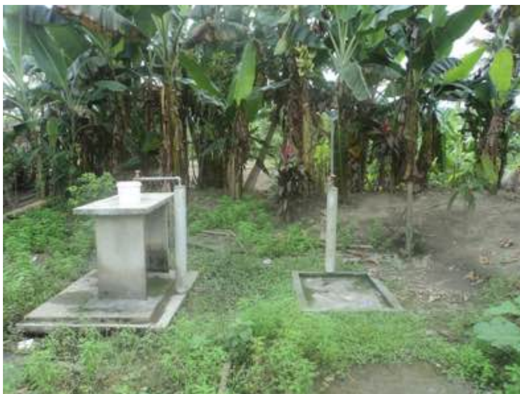
Plate 5.3: Piped water supply in Wongkins village
